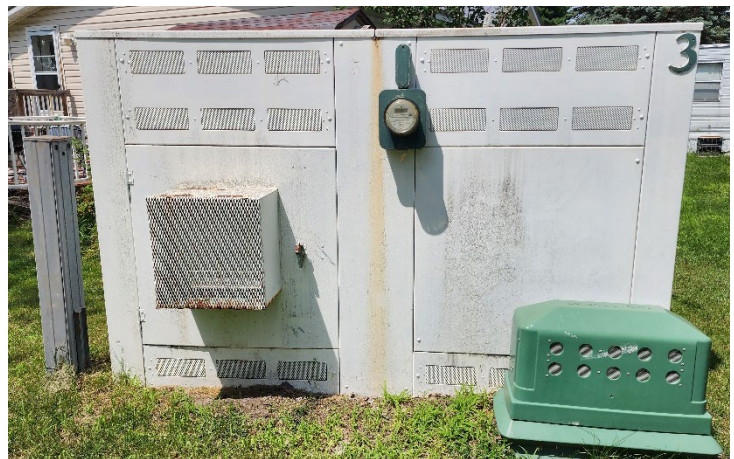
Evergreen Village Aged Transclosure (Polemount Transformer in Cabinet)
