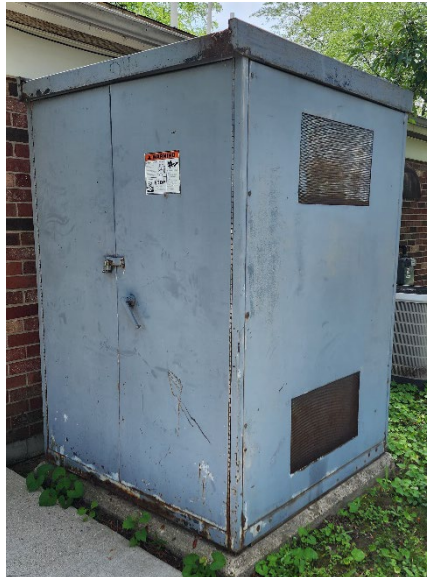
Aged Transclosure (Polemount Transformer in Cabinet)
