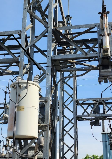
Station Service Transformer
