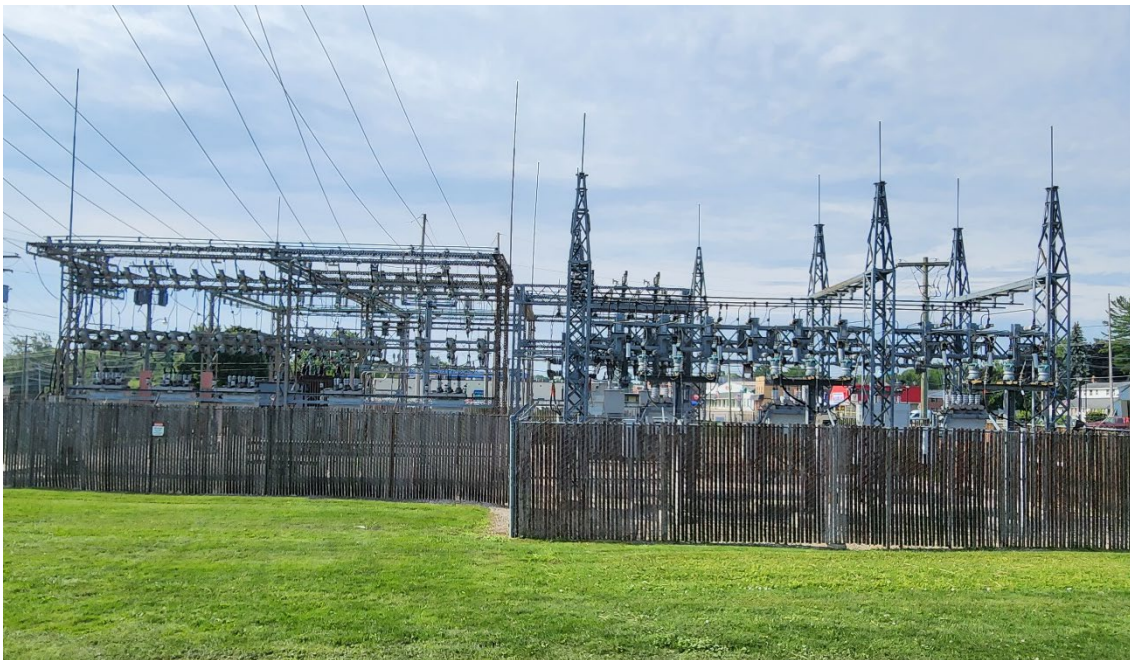
St. Louis / Main Substation City of St. Louis Owned 5kV Facilities
