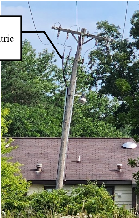
Shepley Apartments Riser Pole
