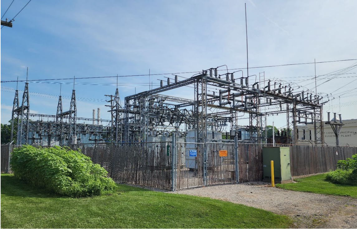
St. Louis / Main Substation Consumer Energy Owned 46kV Facilities
